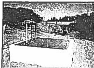
Gate structure in new pipeline. Brownsville Irrigation District, TX.
