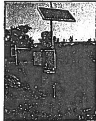
Installation of a solar powered flow meter and SCADA system. Brownsville Irrigation District, TX.
