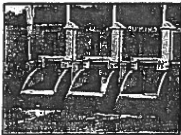
Replacement of manual gates with Rubicon standard programmable flume gate. Cameron County Irrigation District No. 2, TX.
