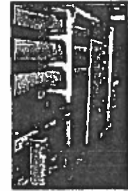
RO energy recovery unit (orange), Naval Facilities Engineering Service Center, CA.
