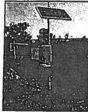
Installation of a solar powered flow meter and SCADA system, Brownsville Irrigation District, TX.
