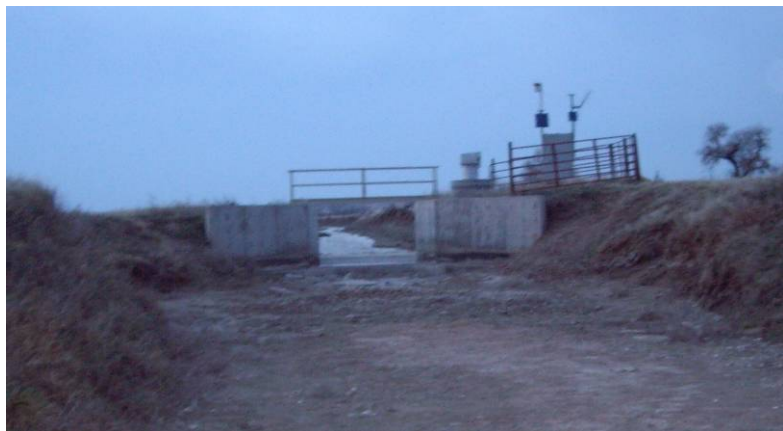
Figure 6.1 South Side Ditch Parshall Flume
