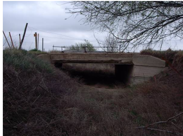
Figure 3.4 County Road Bridge in Need of Repair
