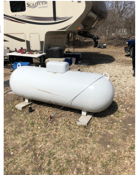
Improperly anchored propane tank
