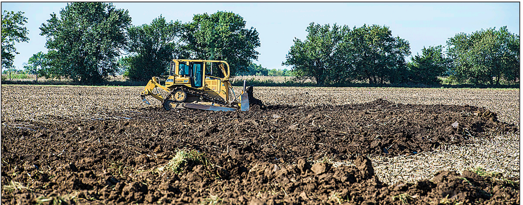
A dozer builds a new terraces south east of Independence. The Montgomery County District helped fund the Terraces with a 50% cost share through Water Resource funding from the State of Kansas.
