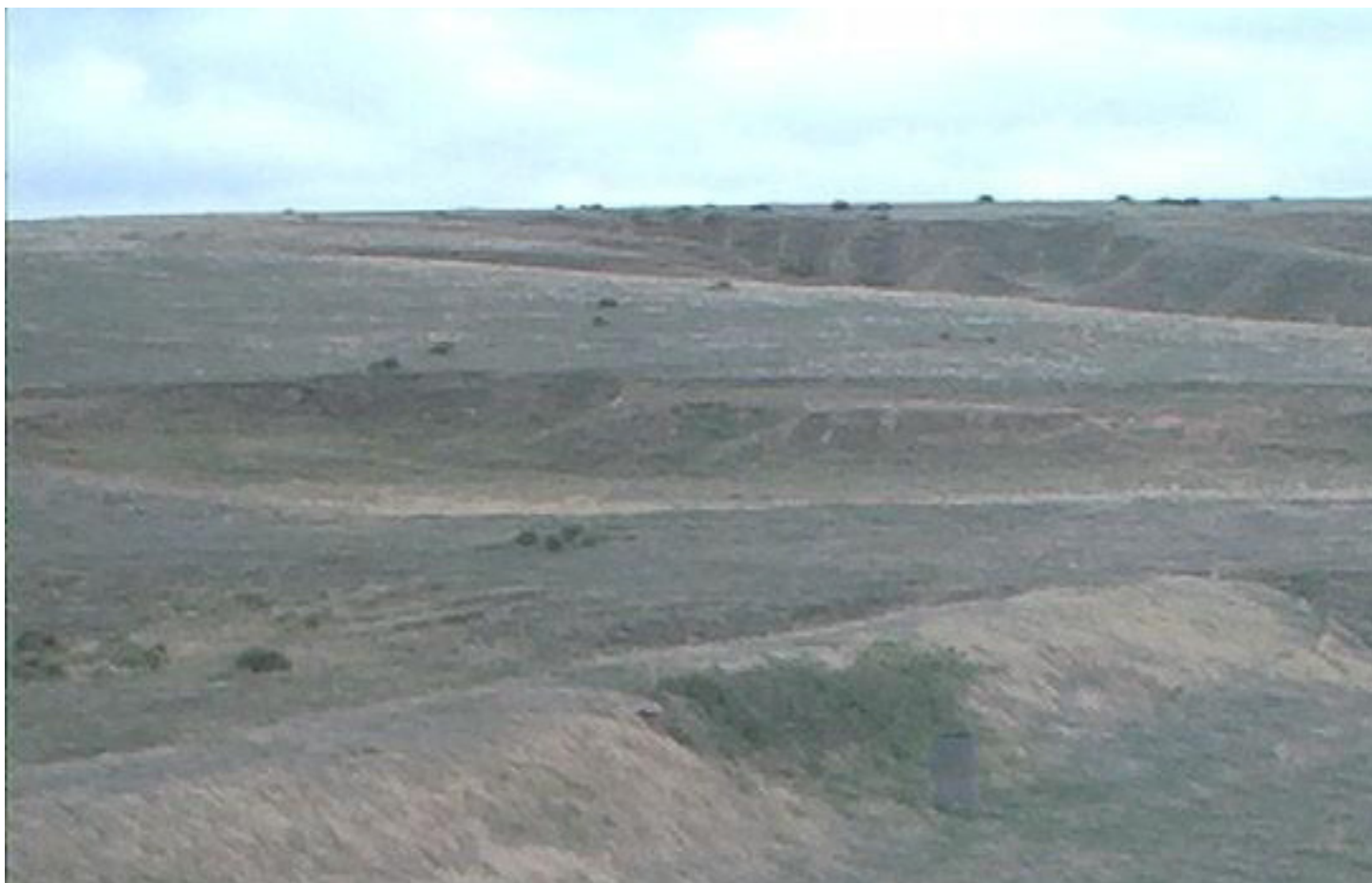
This dam located in western Kansas 350 feet upstream of highway was found to have severe erosion at the outlet of the principal spillway pipe that extended up into the downstream slope and was approaching the crest of the dam.
