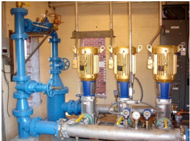
Photo 5 - Example of a High Service Pump Station
