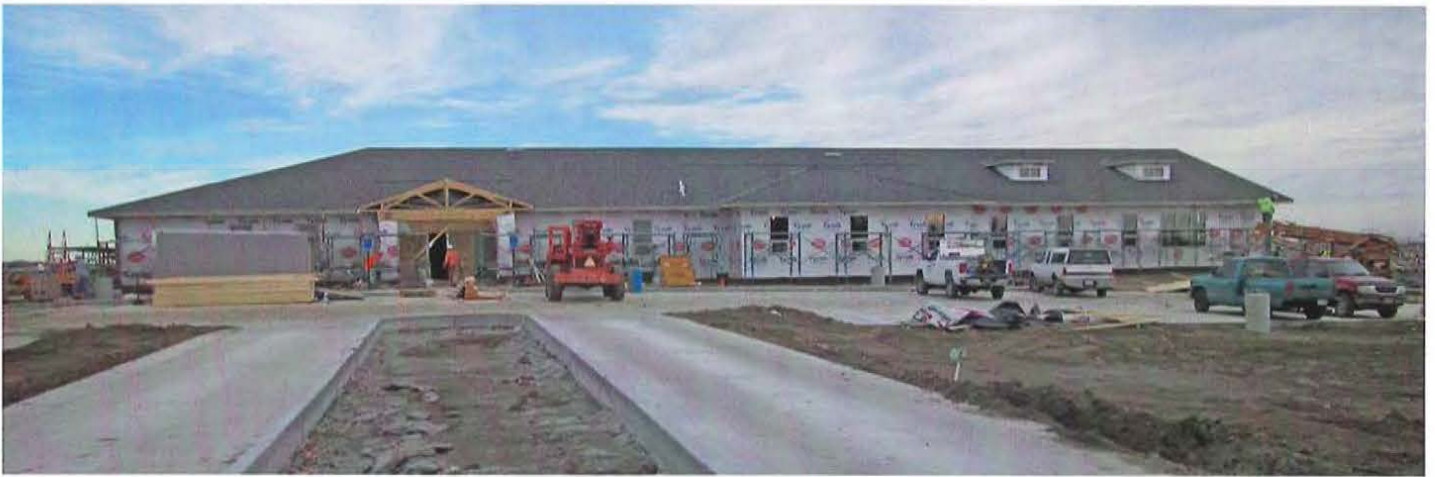
View of new Upper Big Blue NRD headquarters looking north from the paved entrance. Scheduled move-in timeline is mid-March to April 2016.
