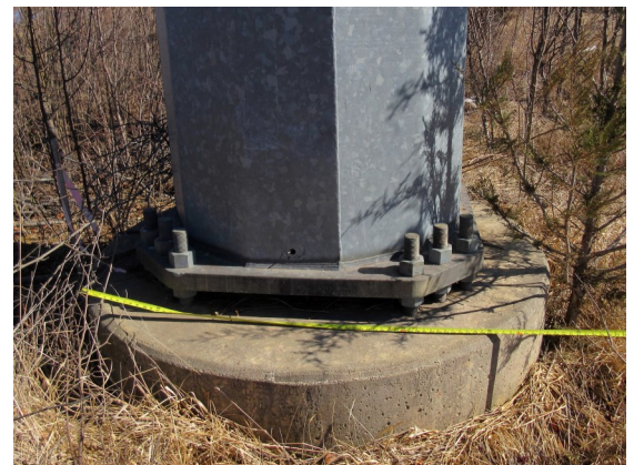
Transmission Pole with concrete base
