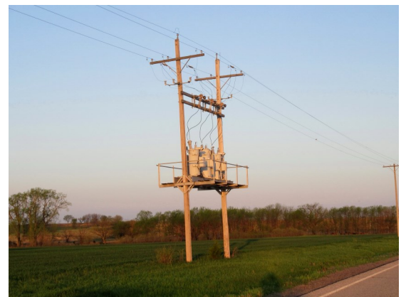
Utilities on platform in the floodplain
