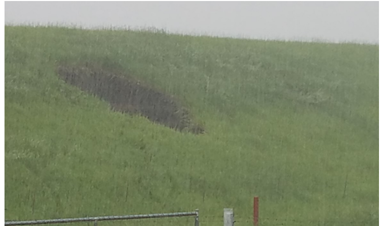
Above: Heavy rain caused a sinkhole to form in a significant-hazard dam near Sabetha, KS in May 2019.
