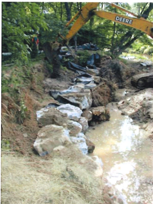
Photo and diagram: A more intensive kind of project our Forestry RCPP may support. Immediate bank stability is achieved by installing stone riprap along the toe of the bank, with channel geometry being modified to provide a low flood-prone surface for energy dissipation. Willows and other flood-tolerant vegetation are established on the low surface, transitioning to shrubs and hardwoods above.
